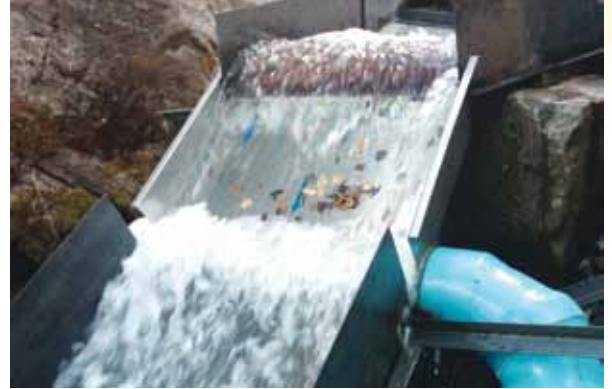
Above: The new intake system at Coal Creek Hydro was installed in October, 2009 in hopes of boosting production and cutting down on manual cleaning. The new system uses self cleaning coanda screens that eliminate the need to scrape rocks and leaves out of the intake valve manually.
