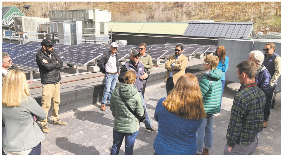
SMPA's Energy Services Supervisor, Phil Zimmer explains the operation of the Telluride middle/high school's battery-backed solar array at the system launch event in April of 2024.
