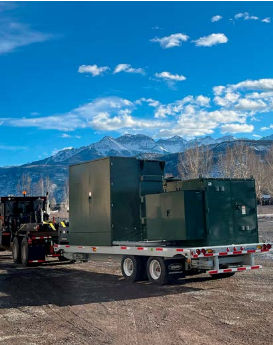
Pictured is the regulator of the Ouray mobile substation. This piece of core equipment, used to distribute electricity to Ouray, is mounted on a large truck-drawn trailer, along with its counterpart transformer [not shown]. Both components provide a secondary system we can rely on while we continue to maintain and upgrade our existing substation.
